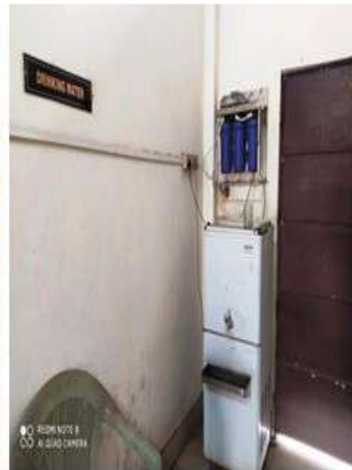
R. O. water filter system
