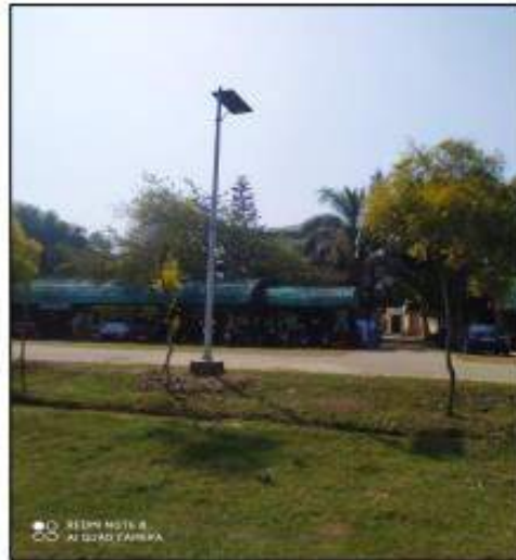
Figure 6. (b) Solar powered Street Light (New Campus)
