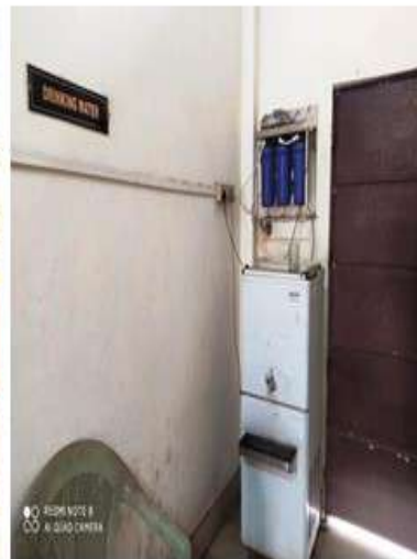
R. O. water filter system
